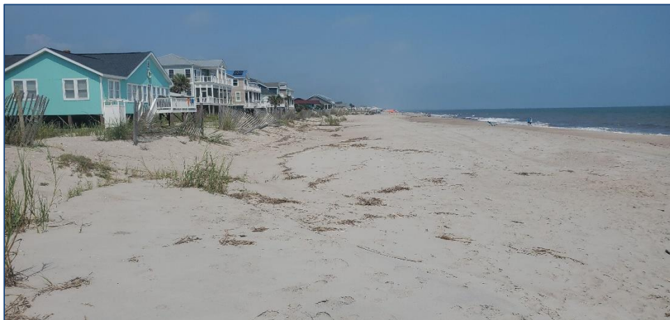
Ground photos of Edisto Beach on 9 September 2019 showing wrack lines at the toe of the dune. Note that much of the vegetation remained in place; however, there was some apparent damage to some sections of sand fencing.
