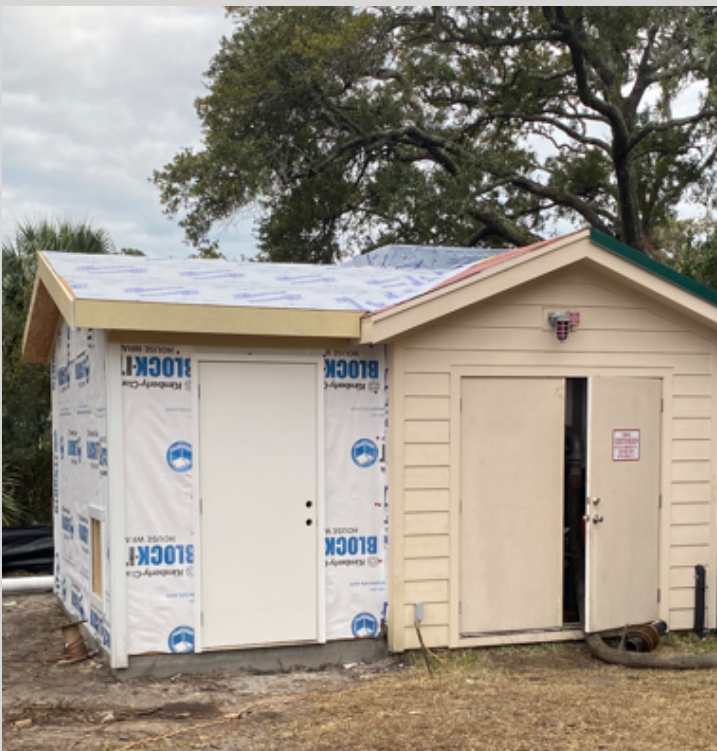
Improvements being constructed to Pump Station B on Gun Bluff Rd. - February 2023
