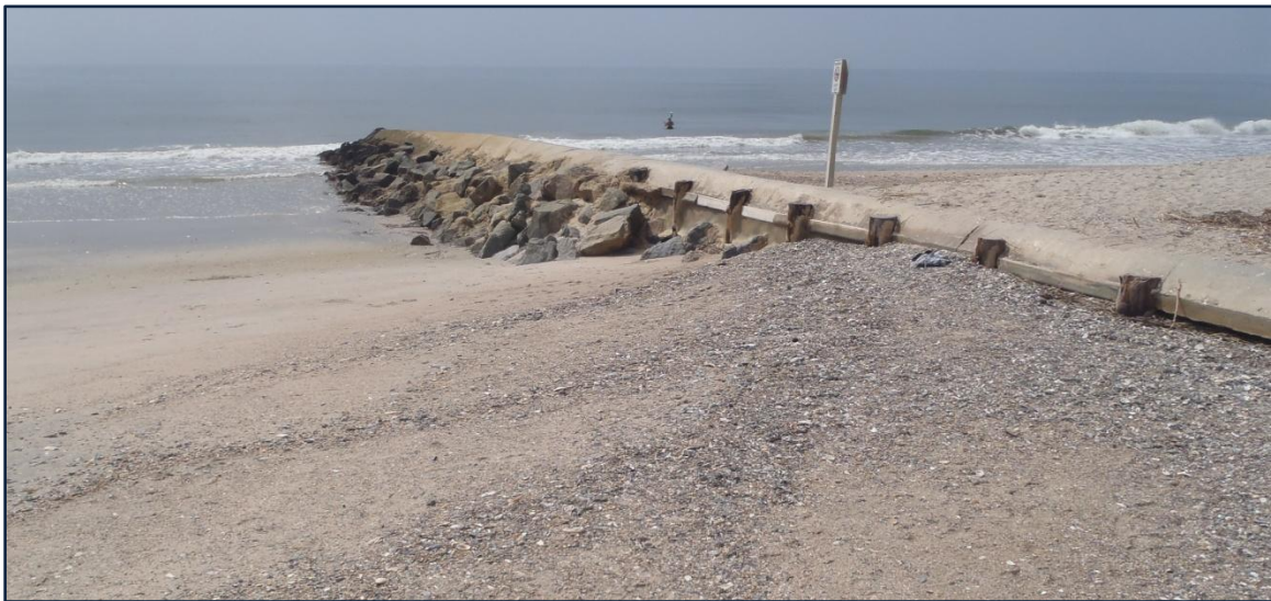
FIGURE 3. Groin 8 at low tide (14 August 2012) showing original timbers (1950s) capped by retrofitted concrete cap (ca 1997). Seaward quarry-stone section was restacked and grouted in 1995. The landward end slopes at ~1 on 50 while the seaward section slopes at ~1 on 20, with the crest terminating about 4 ft above mean low water in this case.
