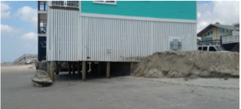
Figure 2. Erosion at Folly Beach caused by Tropical Storm Irene in 2011 and Alberto in 2012, both storms passed more than 100 miles offshore. Photo courtesy of DHEC.
