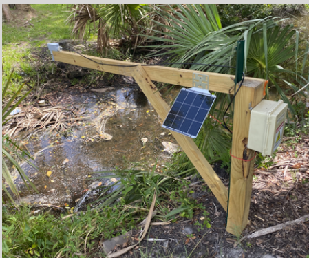
Monitoring station at Nancy Street
