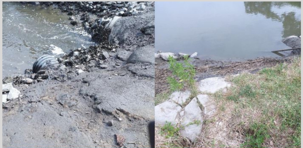
Pictures of the lagoon system outfall to Scott Creek at the intersection of Jungle Shores Road and Whaley Street, which shows the tide elevation change as it approaches low and high points.
