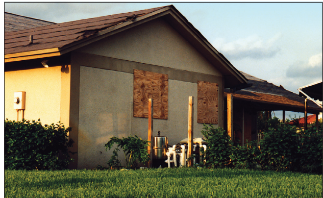
Figure 1. Wood structural panels installed in accordance with building code requirements are a cost-effective means of protection, but they should be adequately attached so they themselves do not become windborne debris.
