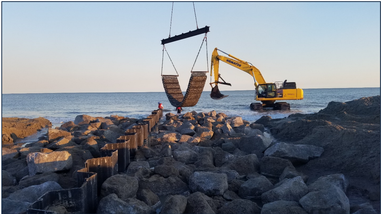
FIGURE 3.8. [UPPER] Installation of UC-95 composite sheets. [LOWER] Installation of marine mattress at the end of a sheet-pile groin.
