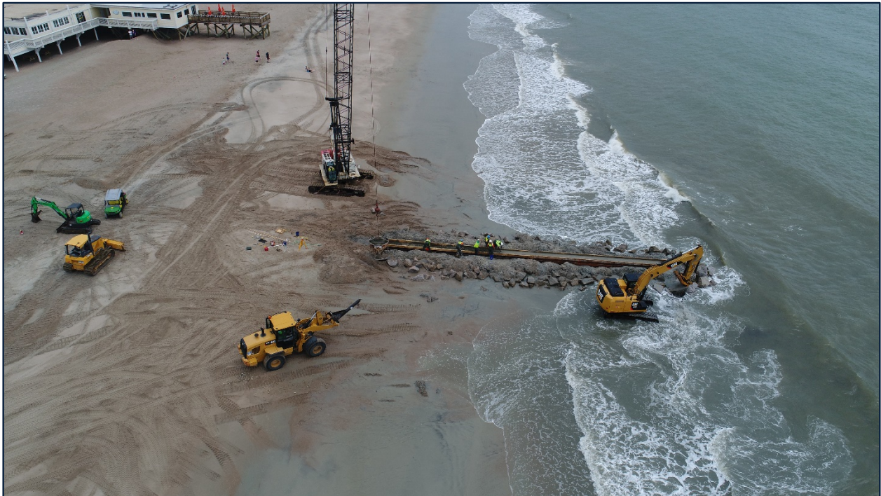
FIGURE 3.9. [UPPER] Pouring concrete into the forms. Note the epoxy-coated rebar (green). [LOWER] Aerial view of groin construction at Groin 2.
