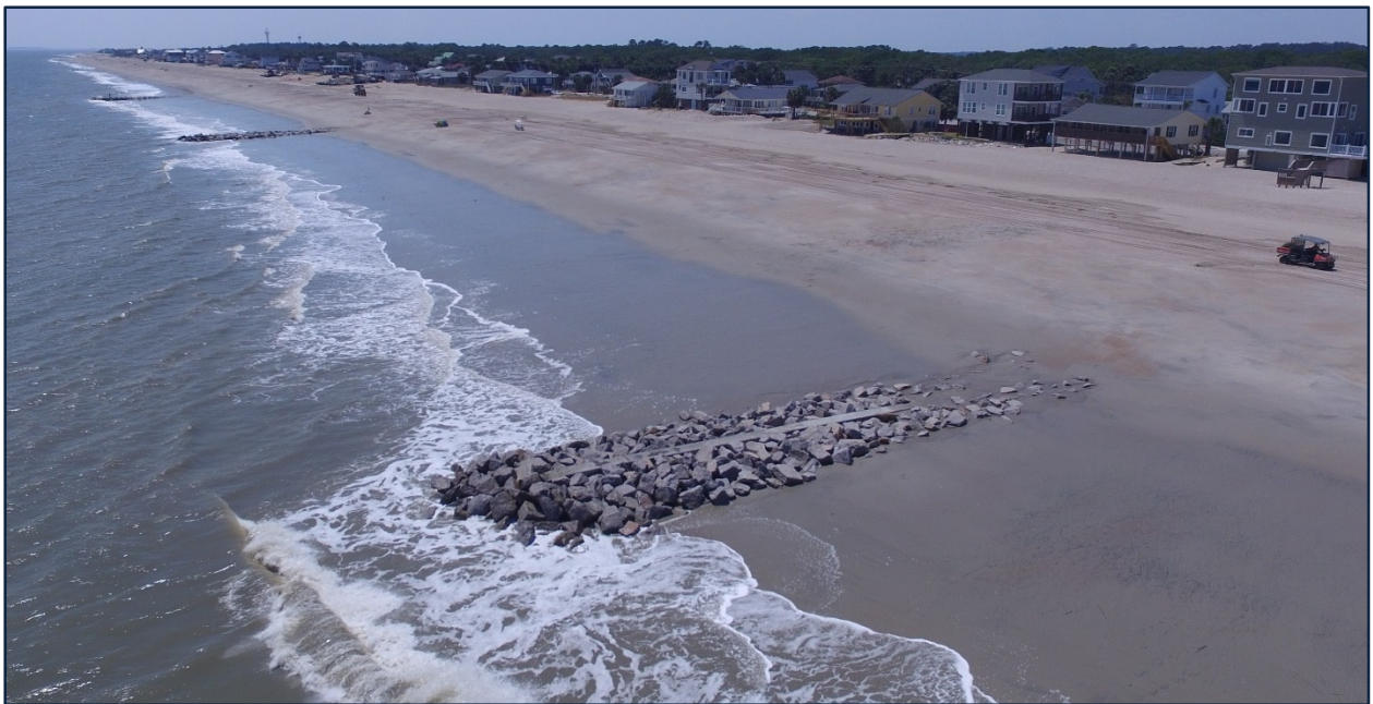
FIGURE 3.10. [UPPER] Pouring concrete cap on the landward end of groin extension. [LOWER] Completed extensions for Groin 7 (foreground), Groin 8 (middle), and Groin 9 (background).
