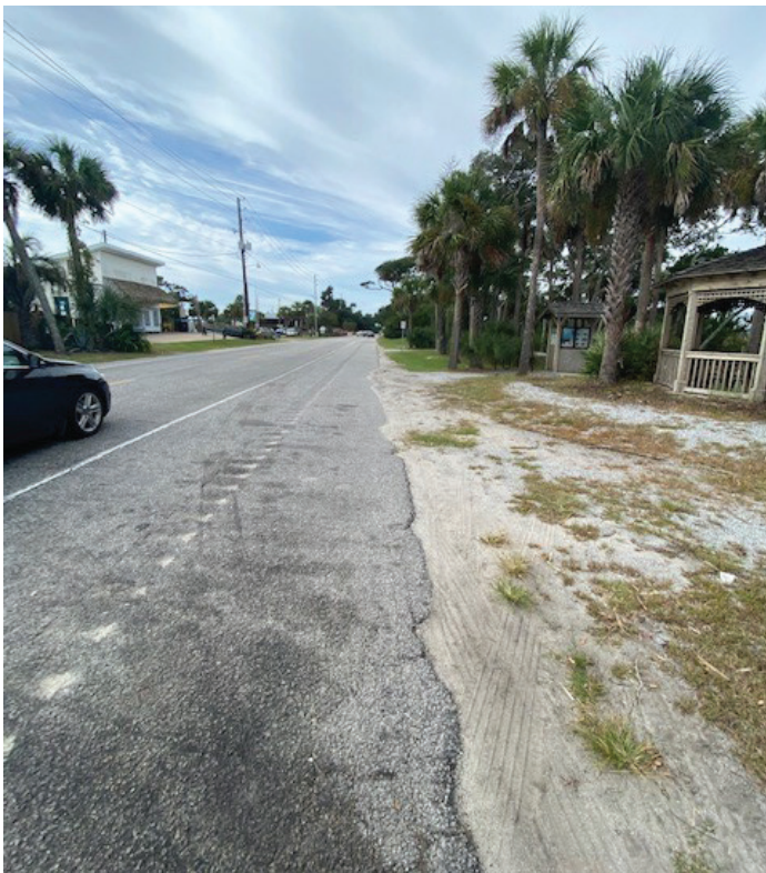
FADED BIKE LANE AT PARK ENTRANCE
